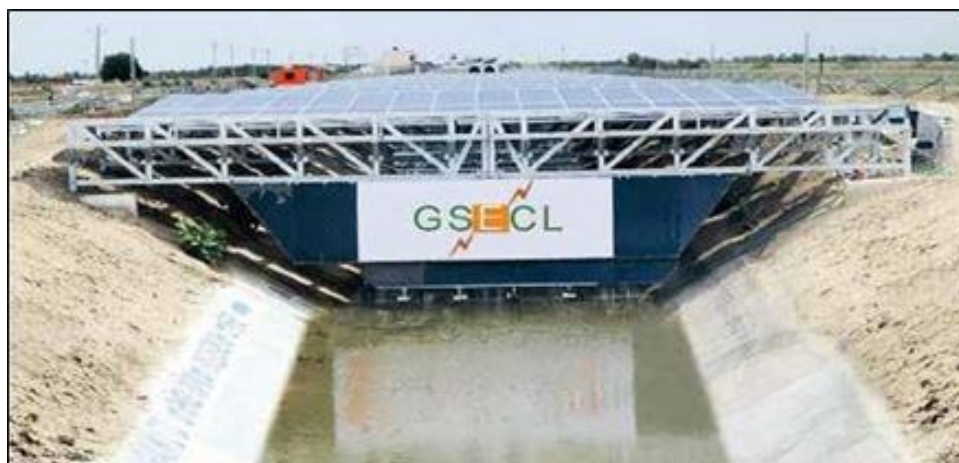
Figure 6: World's first demonstration of canal top solar PV plant at Chandrasan, Gujarat.
