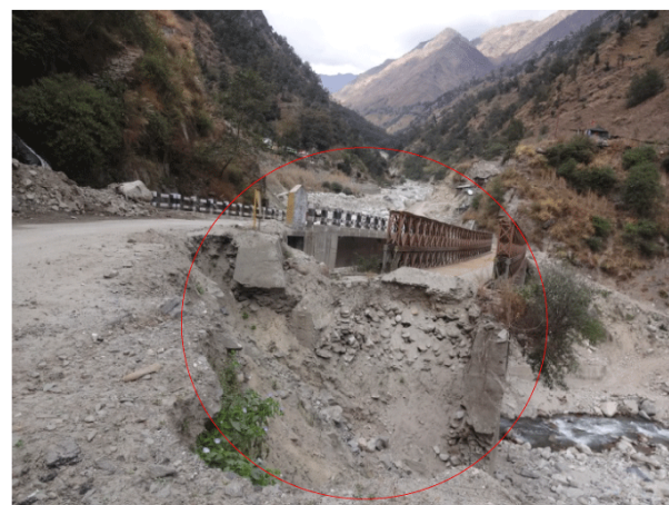
Figure 9: View of damaged right abutment of iron and RCC bridges of Kailash Mansarover Pilgrimage road.
