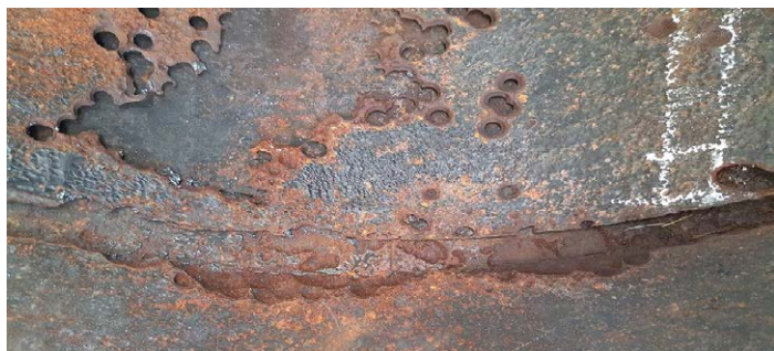
Figure 11: Corrosion morphology in exporting nearby.
