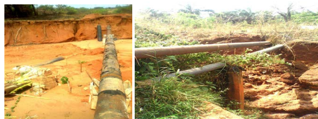
Figure 8: Destruction of Enugu Municipal mains pipes by erosion triggered by mining proximal to the pipelines.
