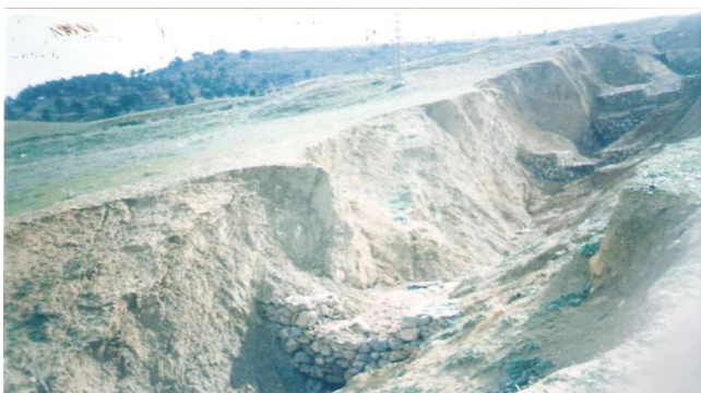
Figure 6: Torrential correction: gabion thresholds Haouch Zegaa - Ouzera shooting 27/03/2007 and at the slope.
