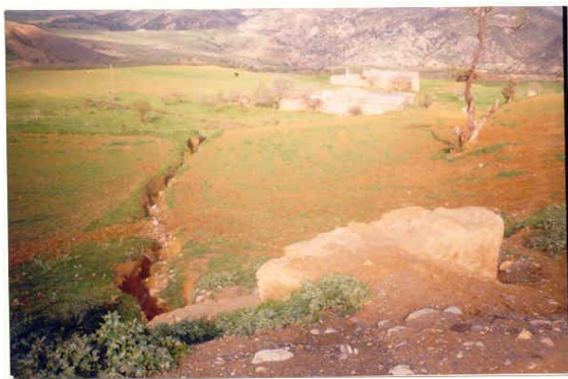
Figure 5: Gully from underground drains all along the road is entering the field.
