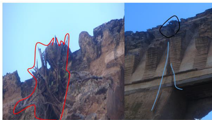
Figure 1: A shows the tree grown on the upper and internal wall of the structure at the south-eastern facade of Adiam Seged Eyasu's Palace and B shows how much the root of the tree (shown at A) go down externally and we can estimate the other part of the root is go deep inside the structure to this much.
