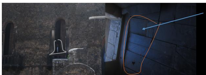
Figure 12: (A) A person standing on the historical wooden structure to have a photo at the back side of the castle of Fasil and (B) The wooden floor of Fasil palace and the circle show the defect of the floor.
