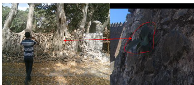
Figure 8: The structure destructed by big trees at Fasil bath and a small tree growing on the left side of the stair goes to the second floor of Fasil palace.
