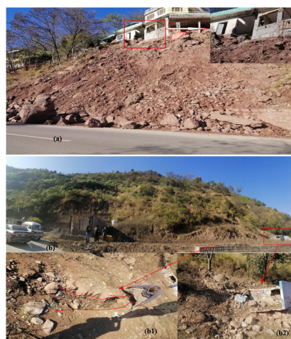
Figure 3: Landslides locations along the Lower Toppa to Kohala Bridge road. (a) Recently damaged local resident's houses by landslide, (b) a large slide happened few years ago caused damage to a petrol pump and few shops ((b1) cracks on the road shoulder (b2) remaining of damaged shops.
