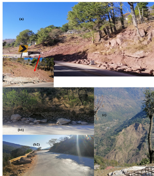
Figure 4: (a) recently occurred landslide's remaining on the left side of road, (b1,2) Damaged retaining wall on both side of the roads due to Rock fall (huge boulders) on the bank of Jhelum River, (c) A massive landslide on the opposite side of the road and left bank of Jhelum River.
