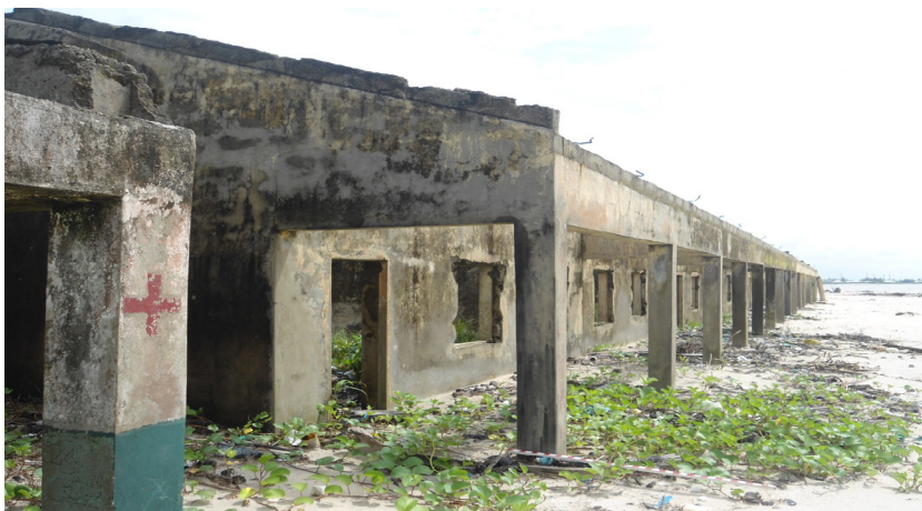
Figure 15: Fomer Itak Abasi Primary school damaged by the storm surge incident in 2011.
