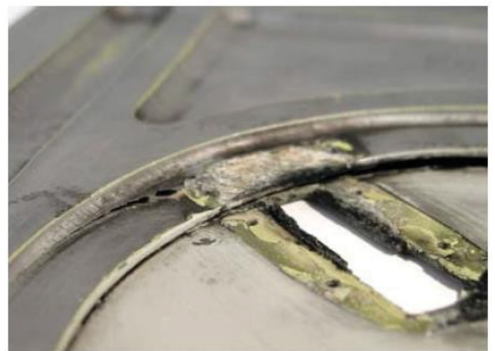
Figure 7: Exfoliation corrosion on inner surface of door and panel around catch position.
