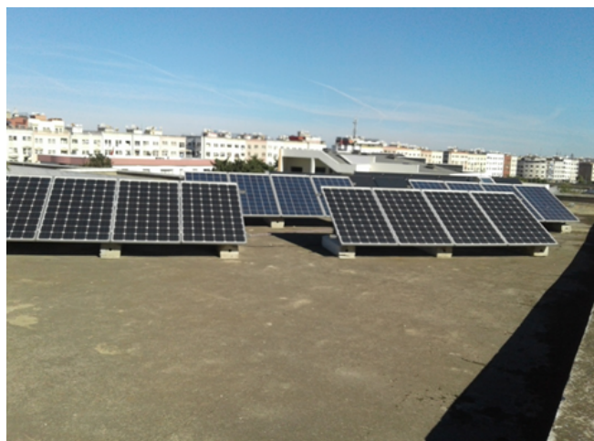
Figure 1: View of 6 kWp PV installed in Casablanca.
