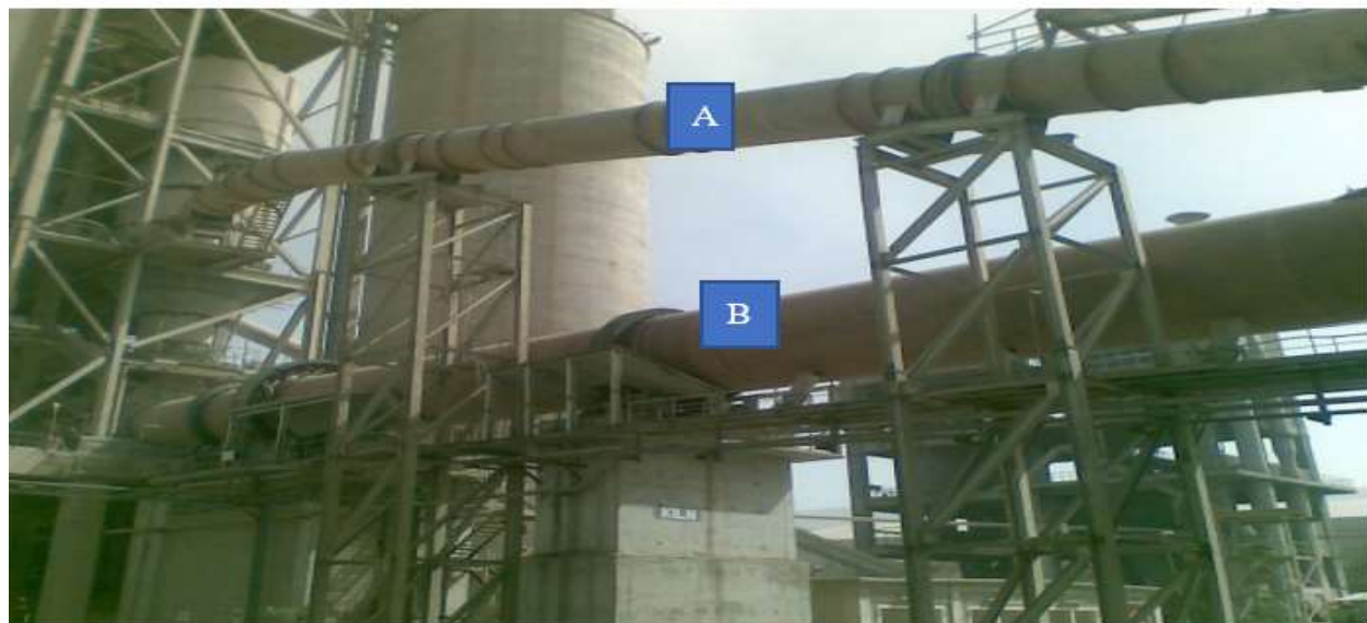
Figure 1: Tertiary duct (A) and kiln of line -I (B) of the company
