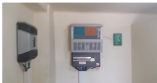
Figure 3: Charge controller and inverter.
