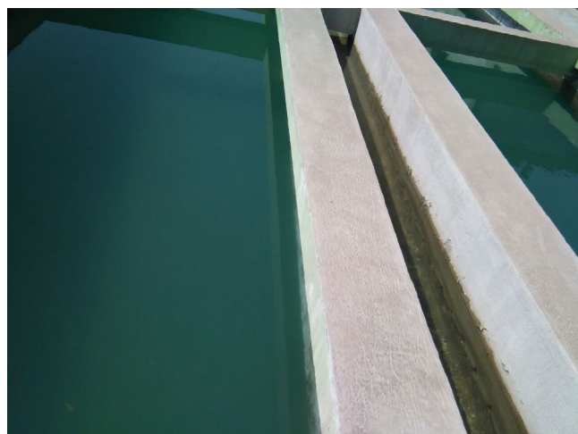
Figure 11: Pluse zone of Pulsator clarifier.
