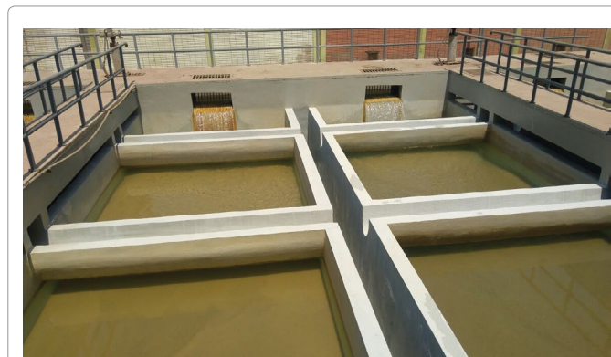
Figure 13: Sand filter with gate inlet and separate drain.
