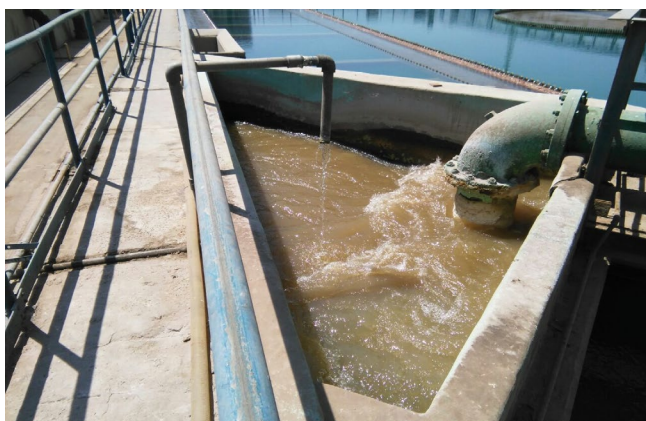
Figure 8: Flash mixing zone in the American and Czech clarifiers.
