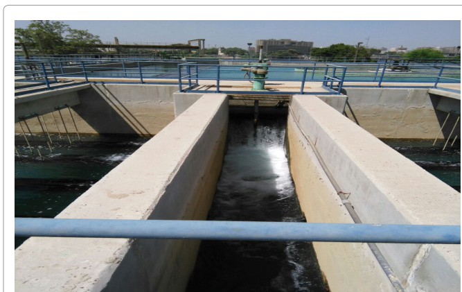
Figure 14: Sand filters with water inlet and waste drain in the same place.
