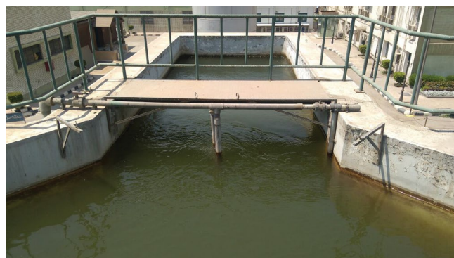
Figure 10: Distribution zone of Pulsator clarifier.
