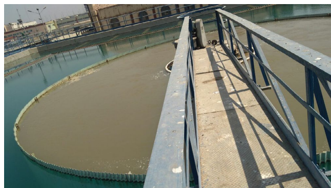
Figure 9: Slow mixing zone in the American and Czech clarifiers.
