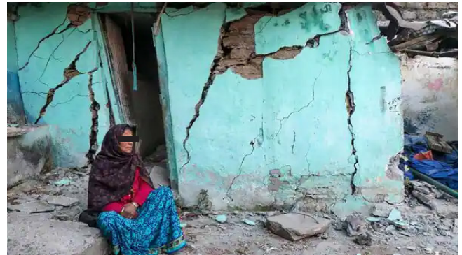
Figure 1: A woman sits beside a cracked wall of her house at Joshimath in Chamoli district (AFP).
