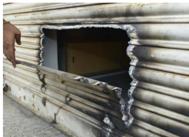
Figure 1: Shutter broken by gas cutter.
