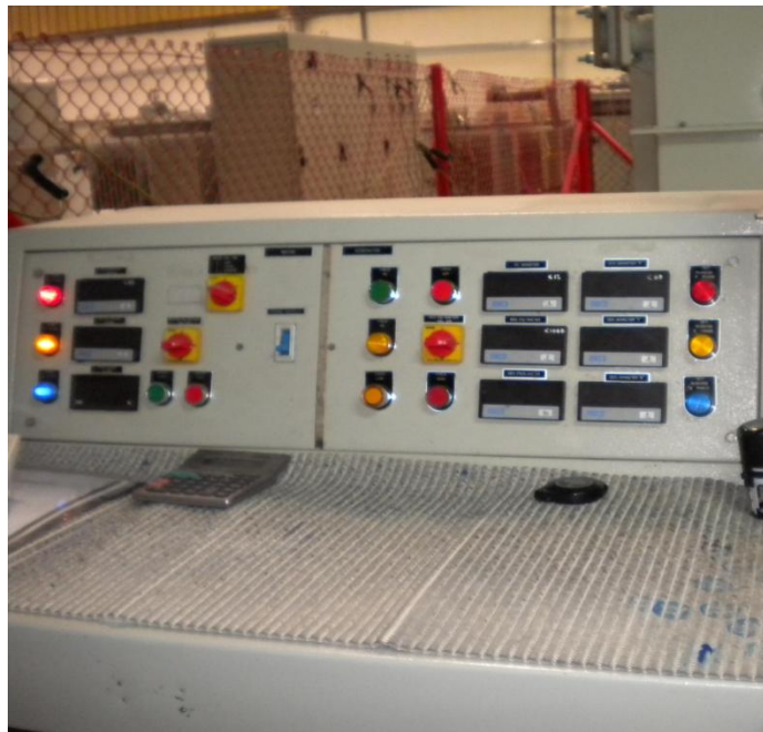
Fig 4.: Induced Over Potential Test Control Panel
