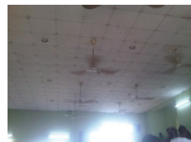
Figure 9a: 600mm x 600mm perforated ceiling boards.
